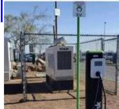
This is an electric charging station, powered by a diesel motor.
